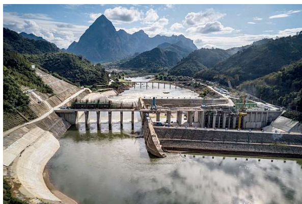
C The Nam Ou 1 Dam in northern Laos under construction in 2018. It was built by China’s largest hydropower company. Sergey Ponomarev for The New York Times
